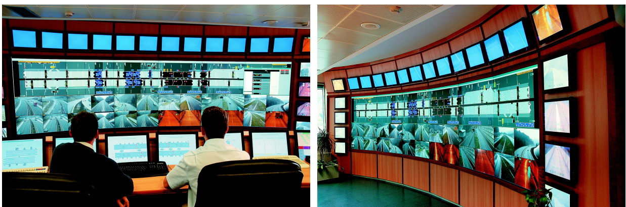
Figure 3: Control room at the Highway Operations and Maintenance Centre Vransko, Slovenia.
